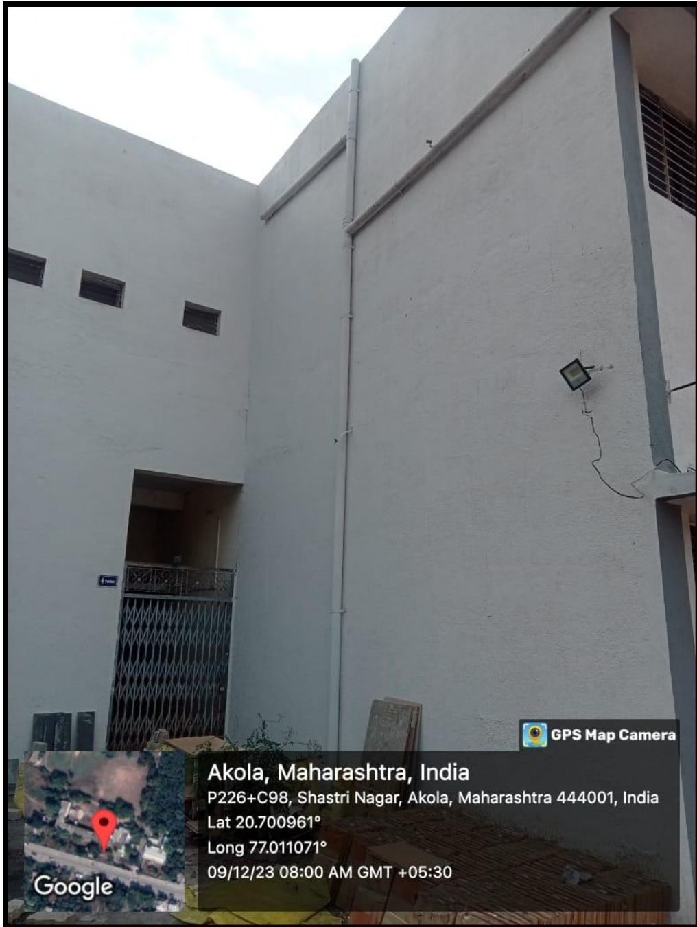
Liquid Waste management – Drainage facility
